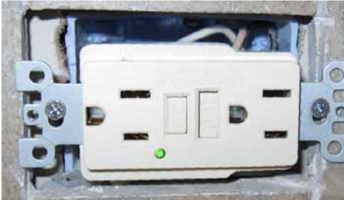
Lack of an appliance box extender
