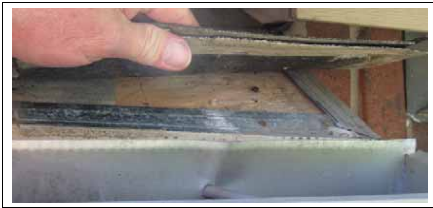
Missing and improperly installed roofing felt
