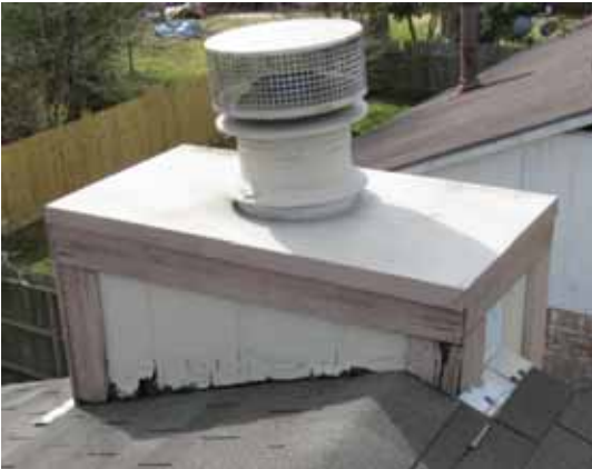
Inadequate clearance above the surface of the roof
