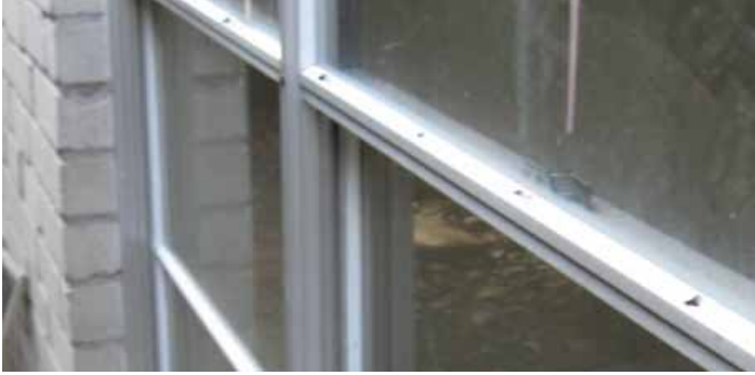
Damaged window glazing strips
