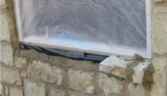
No through wall flashing installed. Water resistance depends on mortar joint. This is an improper installation.
