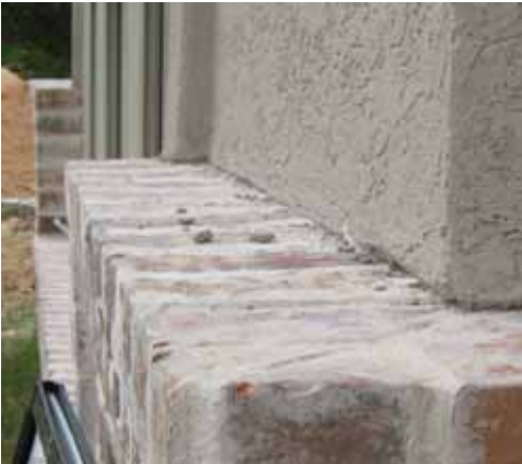
No through wall flashing or drain plane at stucco junction with the brick veneer
