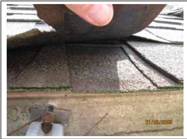
Starter course improperly installed
