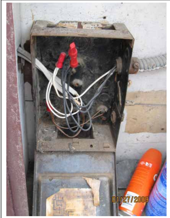
Fuse box used as a junction box
