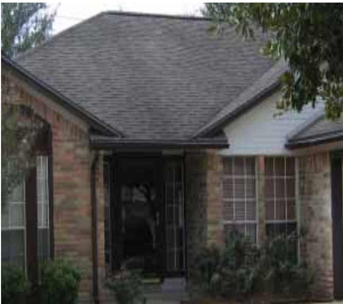
Visible Deflections in the roof Decks
