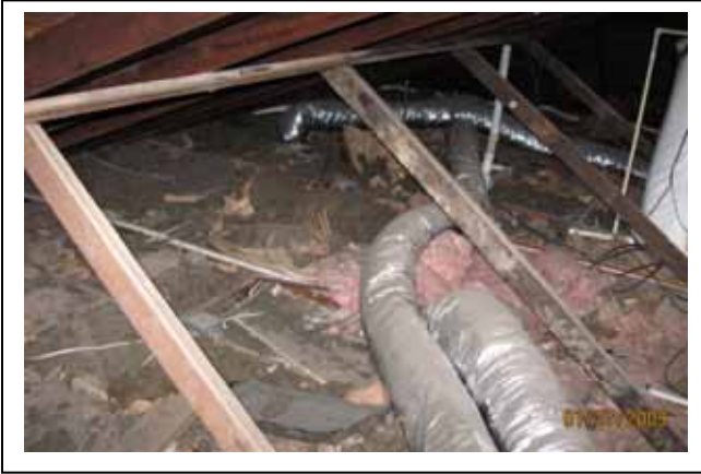
Improperly sloped struts and improperly installed purlin
