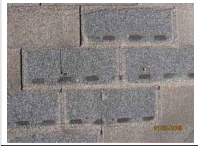
Shingles not properly nailed or bonded
