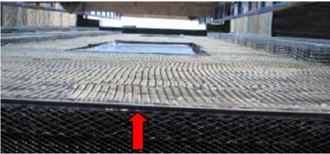
No weep screed or drain opening at vertical wall termination above grade for a stucco, stone or synthetic stone cladding system
