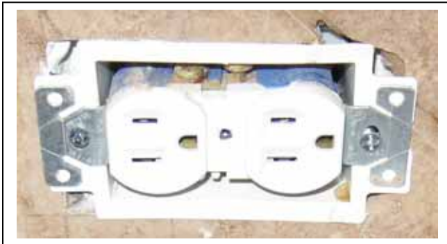
Properly installed appliance box extender
