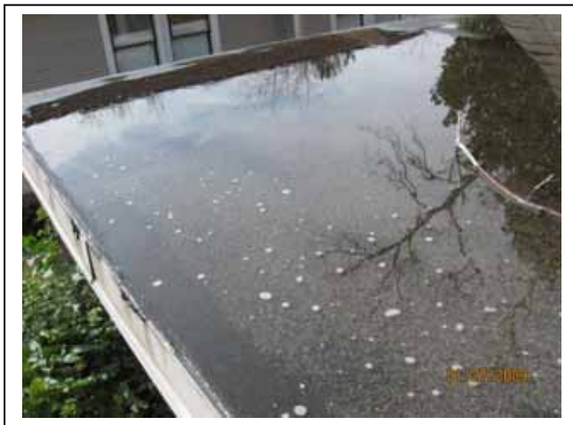
Water standing on a low sloped roof
